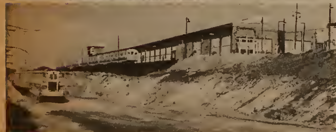
Construction is well underway in all sections of the Corridor. Rail ties and tracks have been removed and excavation of the embankment has begun.
